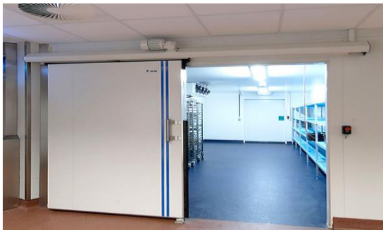
Chiller Cold Room
